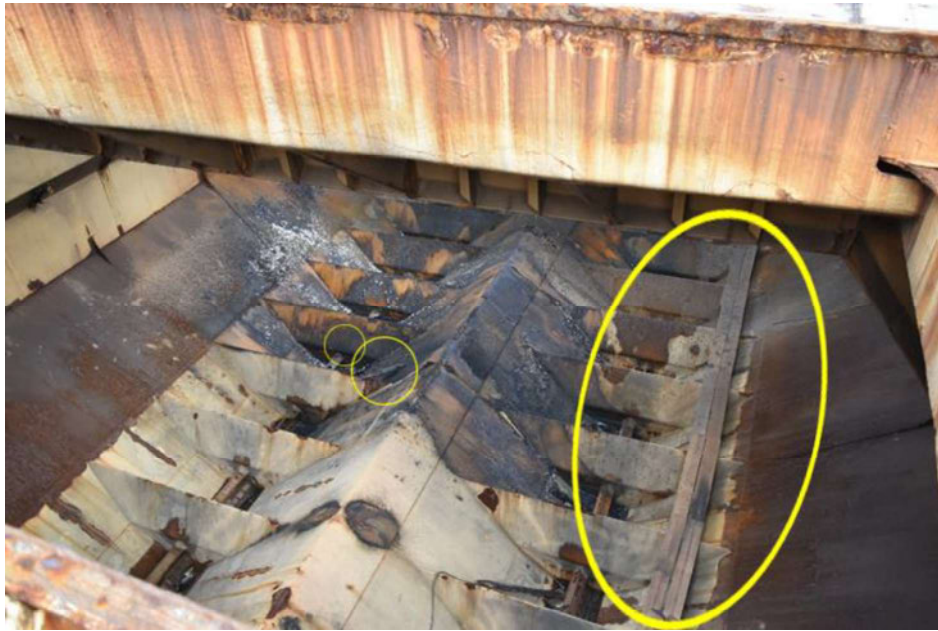
Figure 15. Photograph of charred (portside) and uncharred (starboard side) wood scaffolding planks located inside Cuyahoga 's Cargo Hold No. 2. Source: Ashtabula Fire Department.
